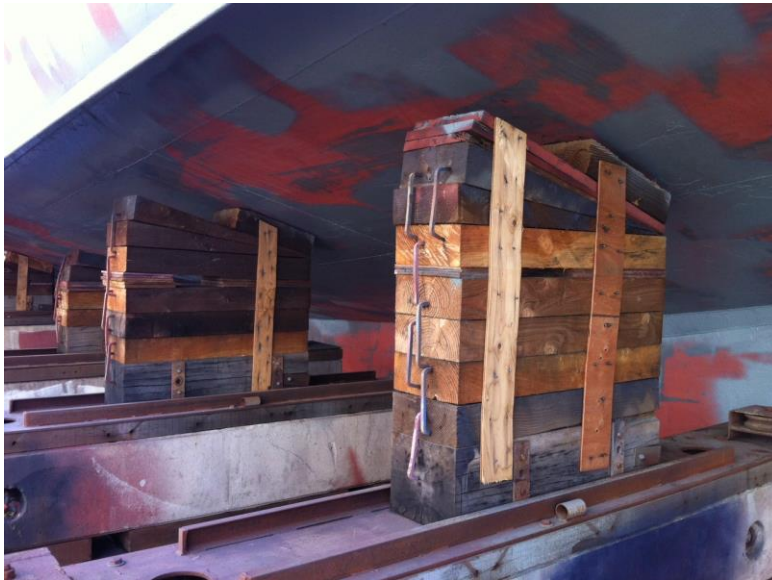
This picture shows current dry dock support system that we intend to replace
